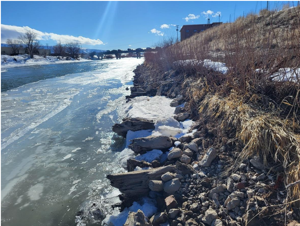
Small erosion area river left sta. 4+25
