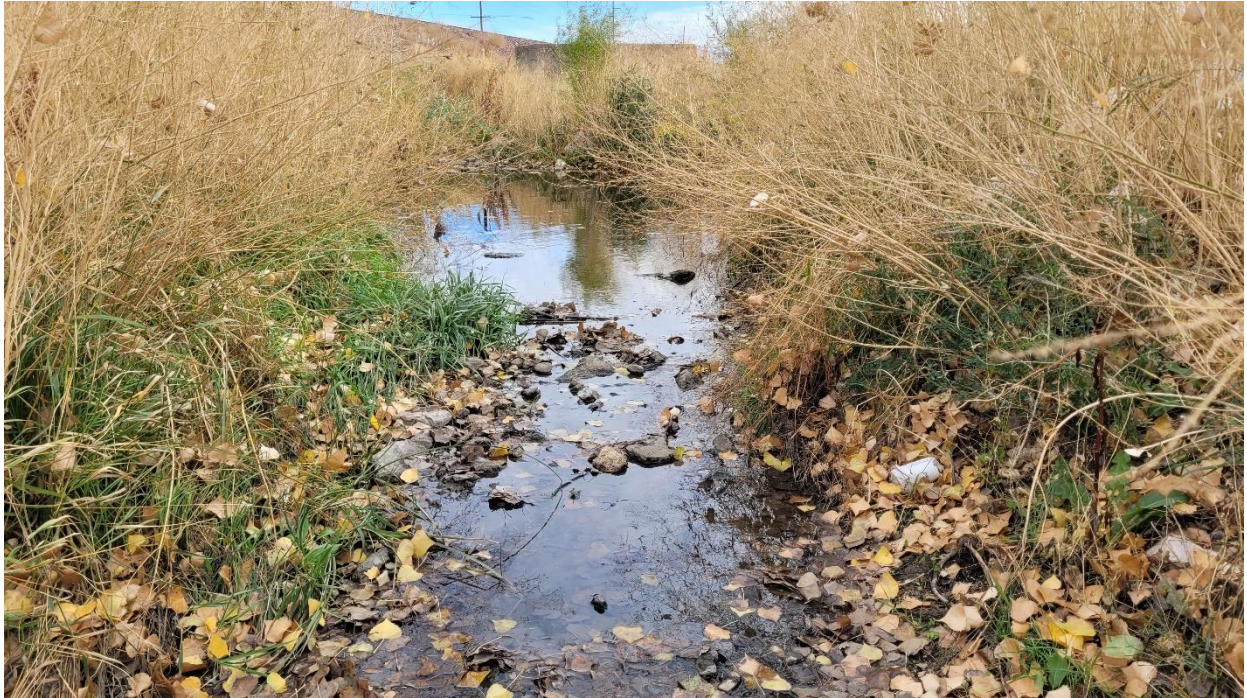
Photo of drainage leading toward wetland from culvert. Culvert is in concrete face just visible at top center of photo.
