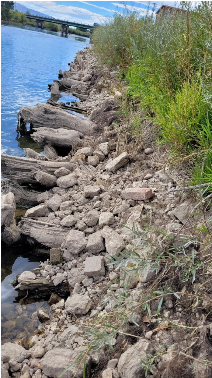
View of woody toe looking upstream, river left, adjacent to Jonah Bank building. Poplar Street bridge visible at top of photo.
