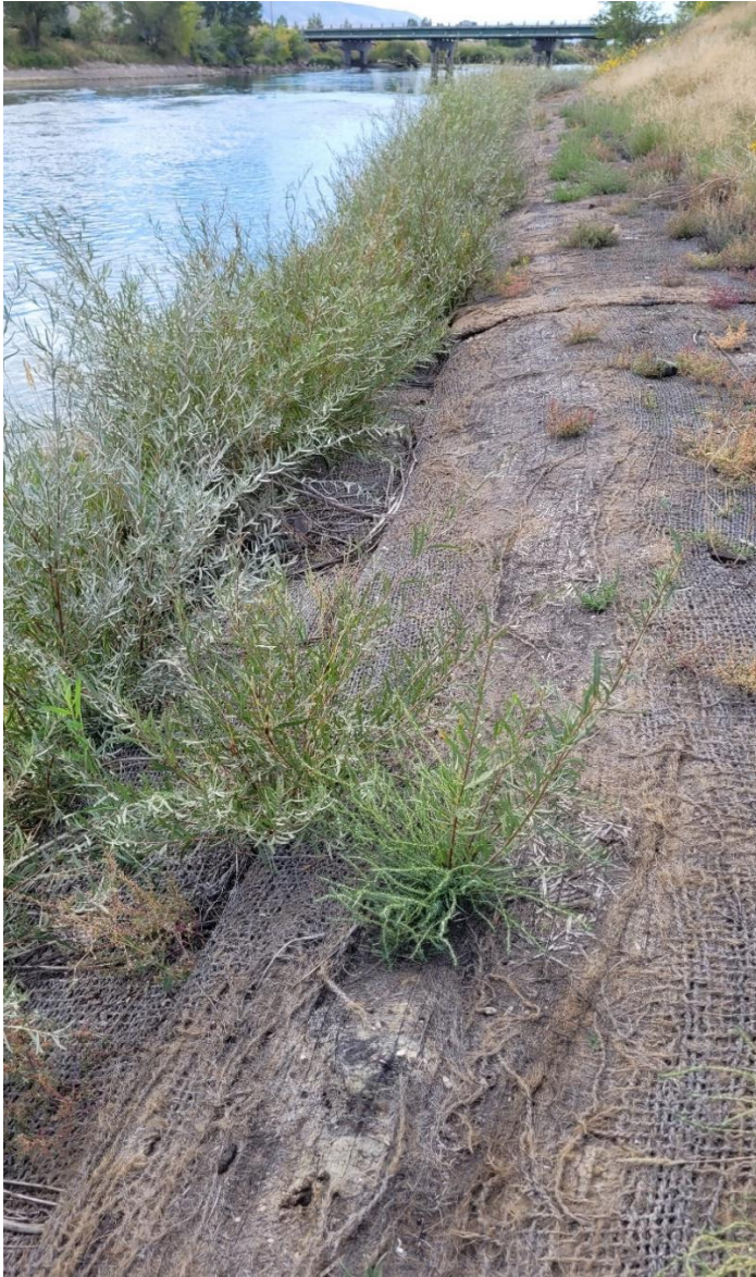
River Left, looking upstream, from Jonah Bank area, Popular Street bridge in upper center of photo. Willow stakes in first burrito established, second burrito rap willow stakes did not grow. Note generally sparse vegetation in second burrito wrap.
