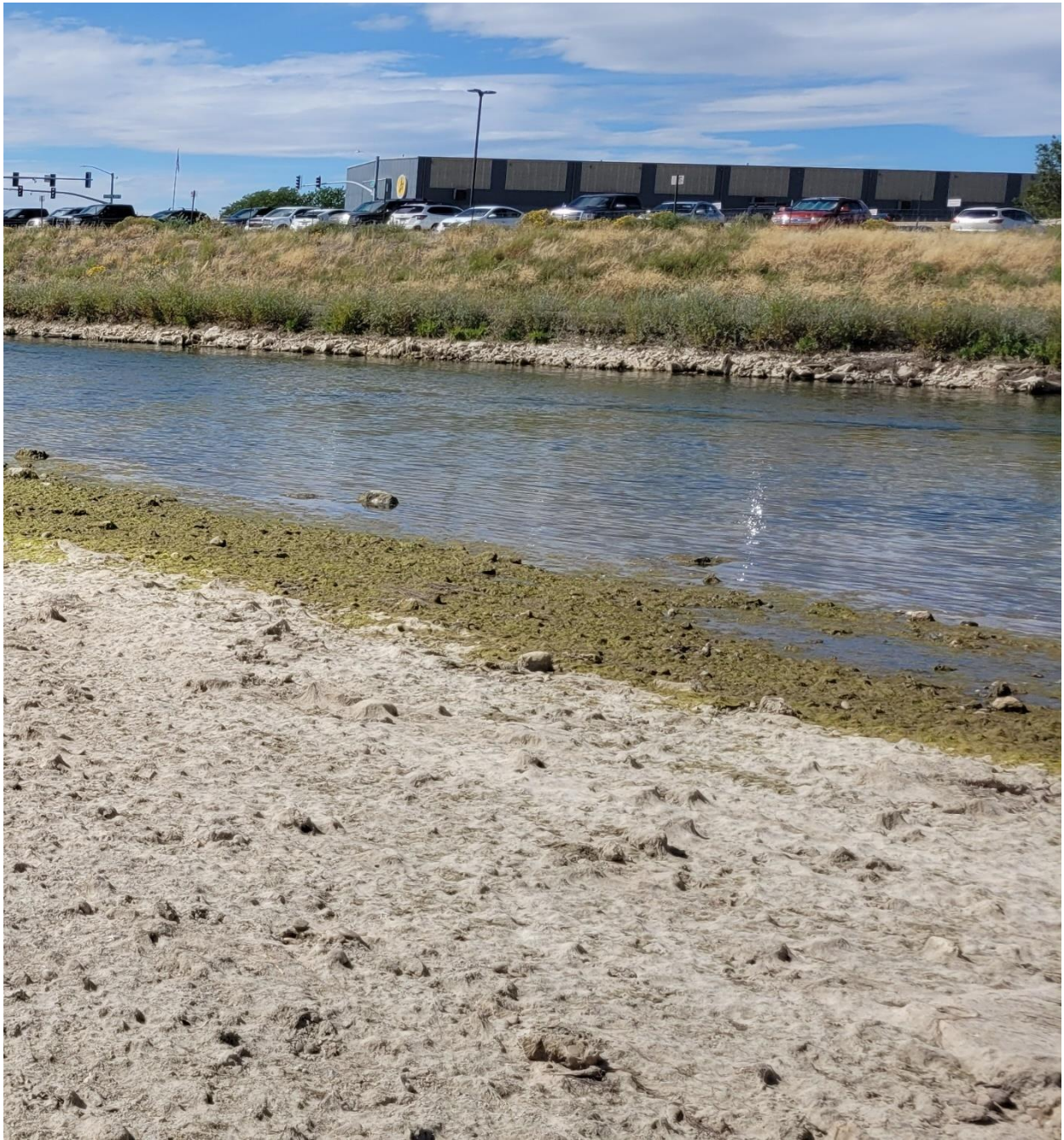
View of river left upper portion of the Jonah Bank area. Note apparent ledge approximately one foot high immediately above the woody toe and cobbles that are exposed due to lower river level.
