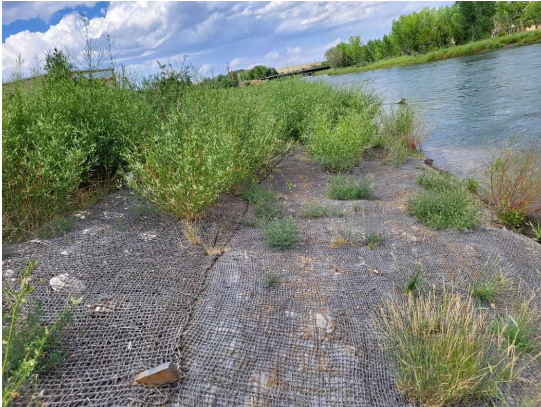
River left from sta. 13+00 to 15+00, more than 70% coverage with a majority of all growth being weeds
