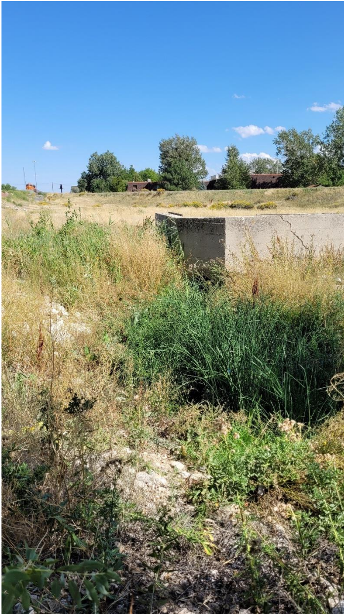
Photo of drainage leading toward wetland from culvert. Culvert is in concrete face top right of photo.
