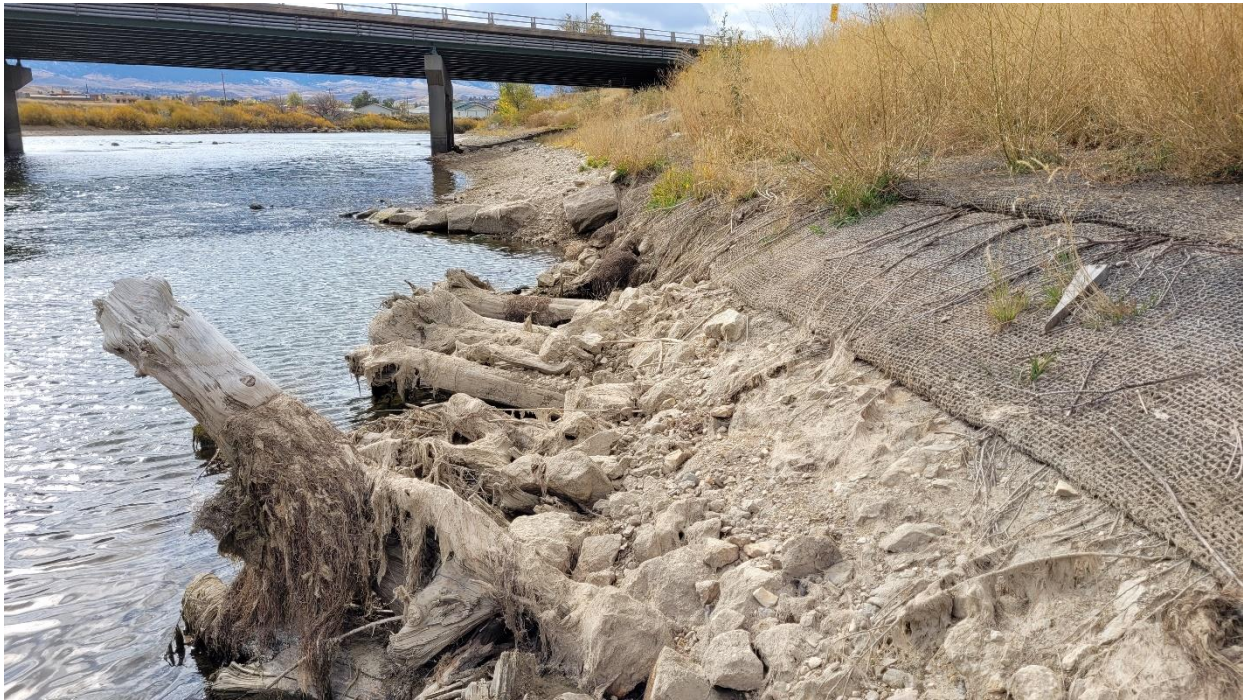
Downstream of 1 st Street Bridge, looking upstream, river left. Note slight indent just downstream (below) of boulders extending into river, with bank steeping due to local bank erosion. Monitoring well cluster is just out of sight in upper right of photo.
