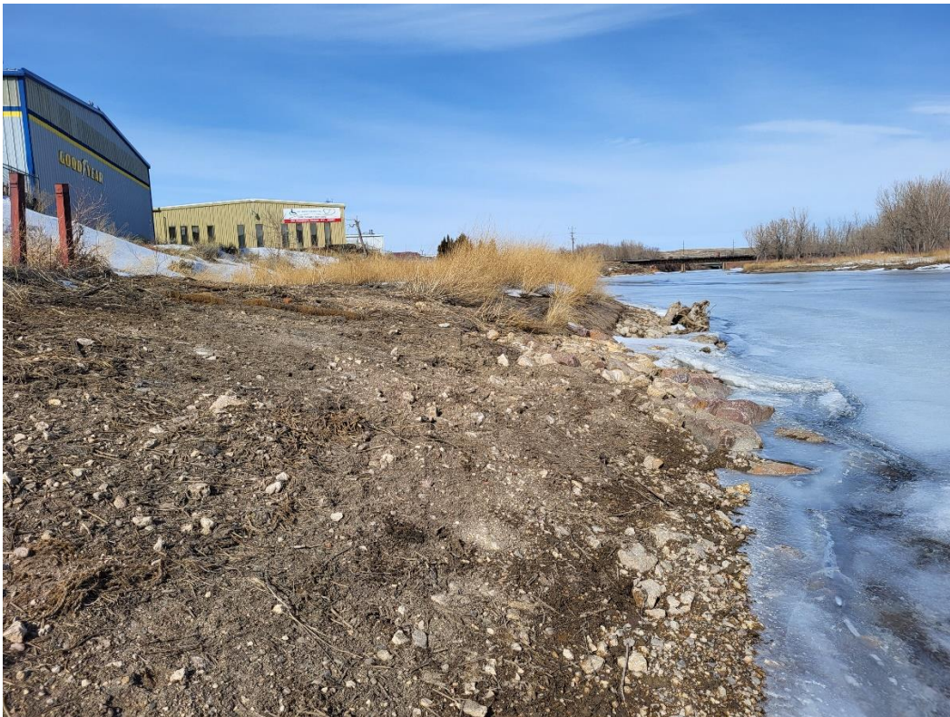
Recently repaired erosion area river left just down stream from First Street Bridge
