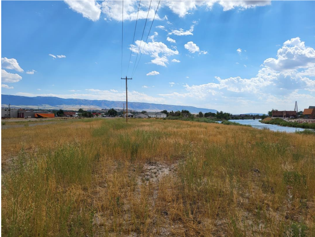
Vegetation in the contractor's staging area has reestablished to 70% coverage or better
