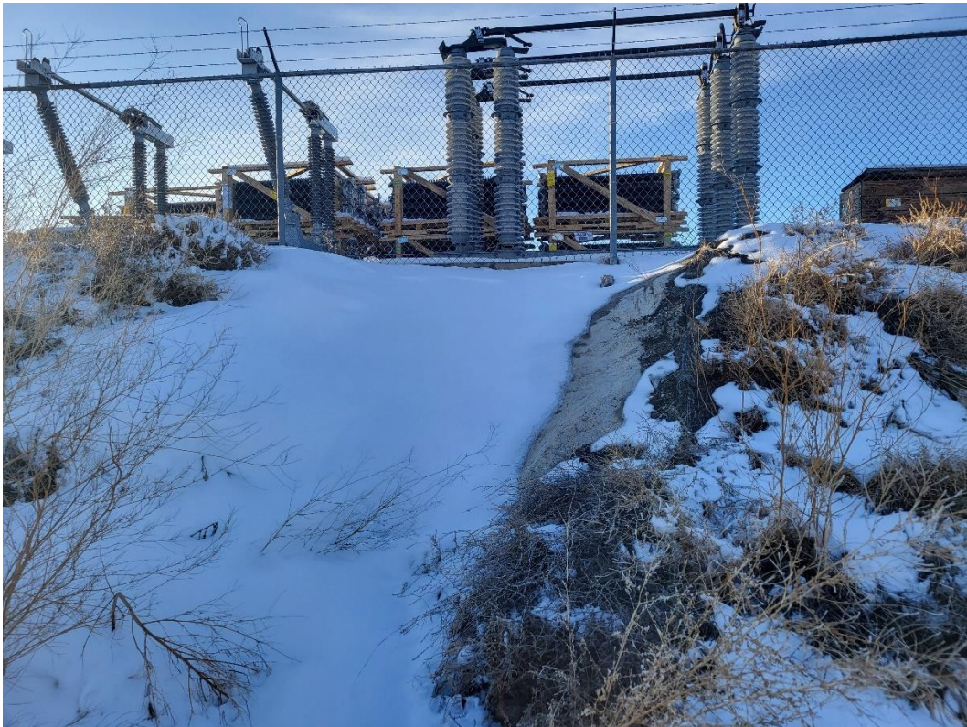
River left, erosion area on the back of the utility yard. A concrete apron was added to this area. Watch for erosion to occur past the concrete apron
