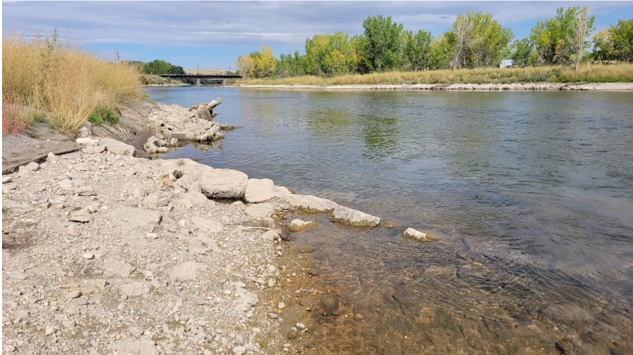
View of river left, slightly downstream of 1 st Street Bridge. Note what appears to be a short distance of bank erosion between rock structure upstream and woody toe downstream. This is not readily visible at higher river levels.
