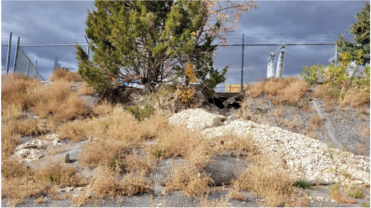
Bank erosion noted in previous inspection, in area of power company yard. Note relatively sparse vegetation, less than 70% coverage overall.
